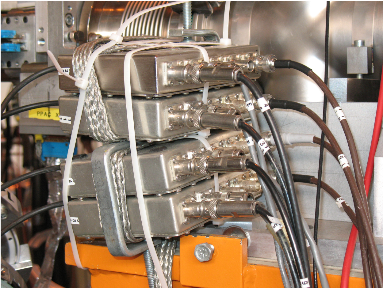
Figure 6: The preamps for the PAD detector which are clamped at on the beam line at the downstream end of the target chamber.
