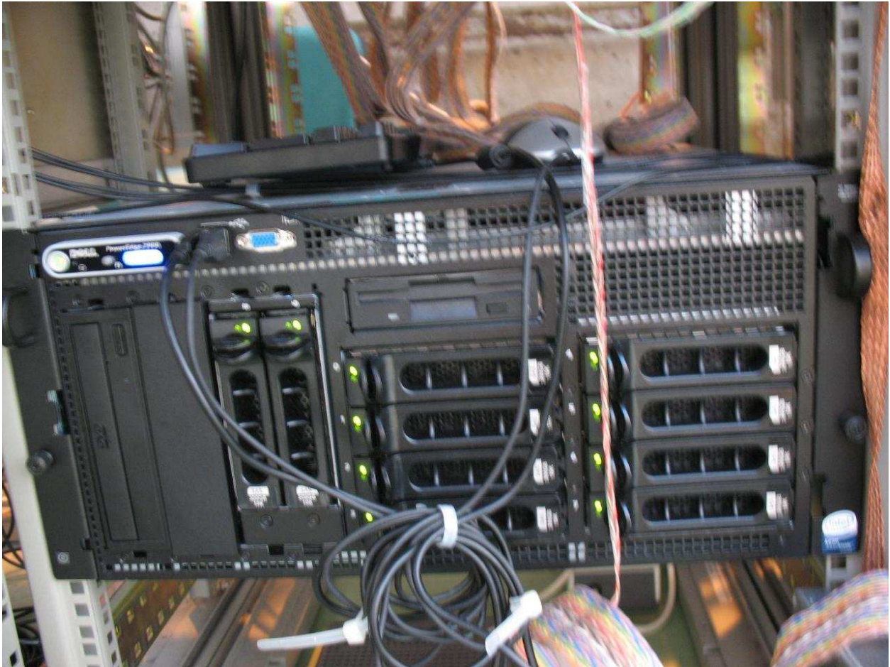
Figure 24: R2.C3: The new DAQ computer and raid array
