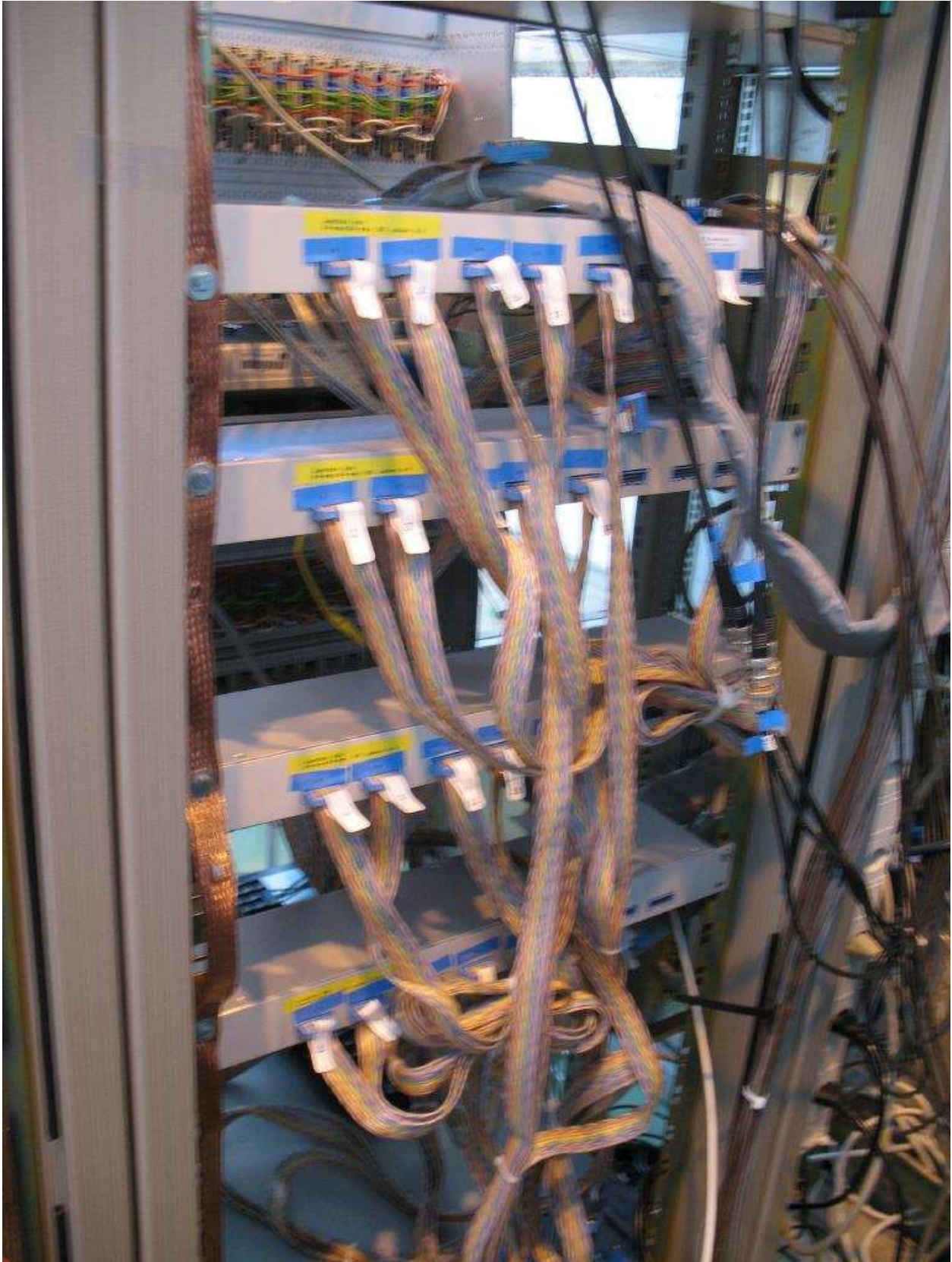
Figure 25: R2.rear: various CD connectors and power supplies
