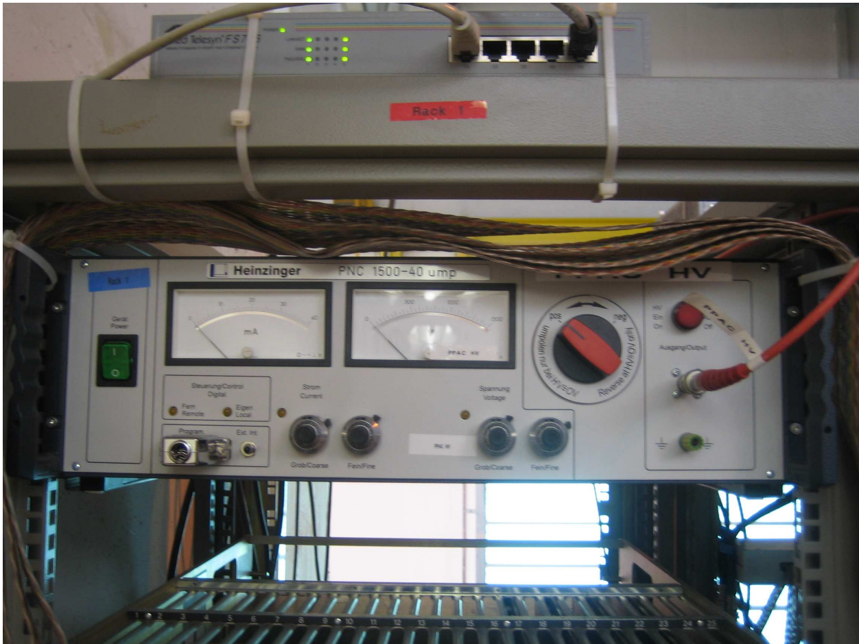
Figure 20: R1.C1: PPAC power supply. We normally use about +400 Volts
