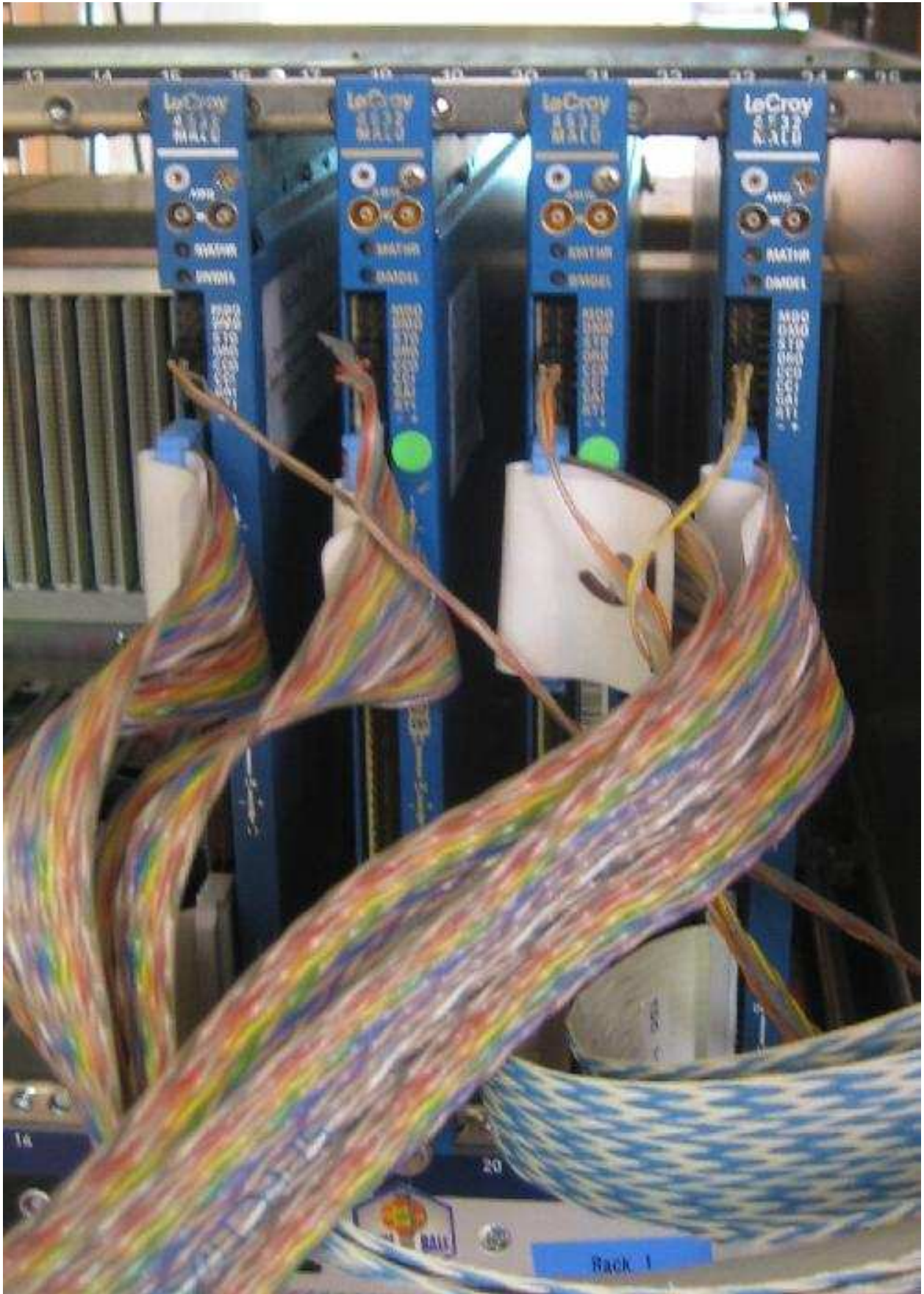
Figure 21: R1.C2: The cabling of MALUs - four multicoloured flat cables (one from each quadrant - the other ends are split in pairs, so they go to 8 RAL109s) come from the RAL109s in R2.C2 (i.e. the front rings) to the inputs. Four blue and white flat cables go from the outputs of the MALU to the TDCs. The ORO output of each MALU goes to the ECL→NIM converter (R2.C3.S1).
