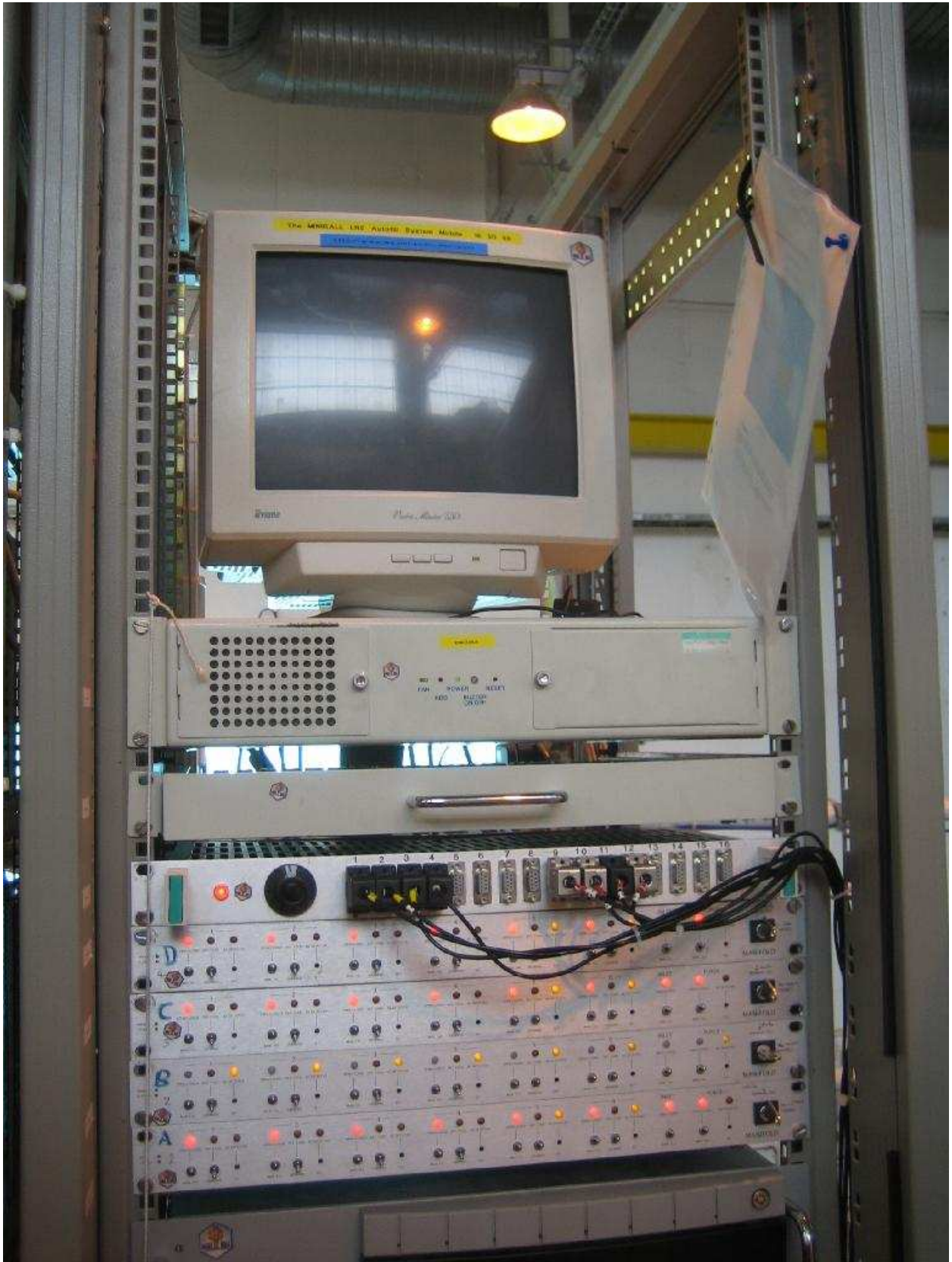
Figure 33: R5 top: filling system computer with monitor and keyboard, PT100 box and four manifold controller boxes.
