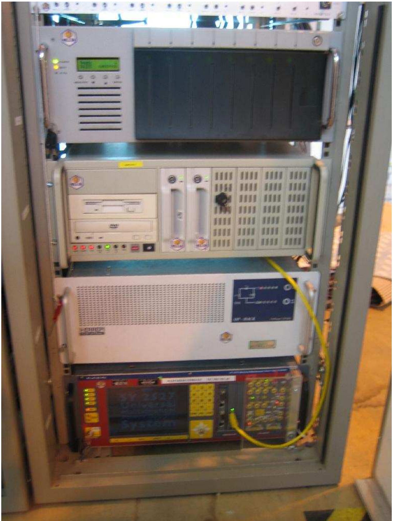
Figure 34: R5 bottom: Raid array, DAQ computer, UPS, CAEN HV power supply.
