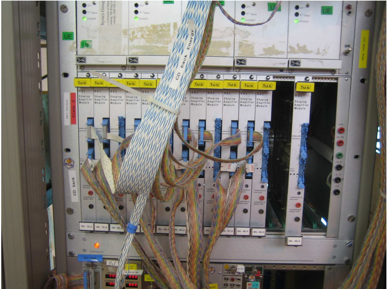
Figure 23: R2.C2: The RAL109s for the back sectors. The upper connections are for the energy and they are joined up in pairs and sent to the ADC. Note that the first pair has the blue and white cable on to which the signal for laser power is added. The lower connections are for the timing and they go directly to the TDC in R3.C1
