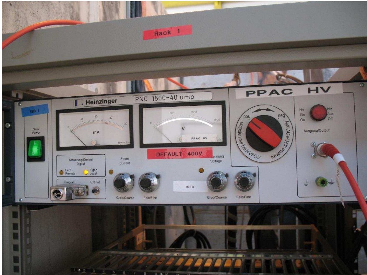
Figure 24: R1.C1: PPAC power supply. We normally use about +400 Volts
