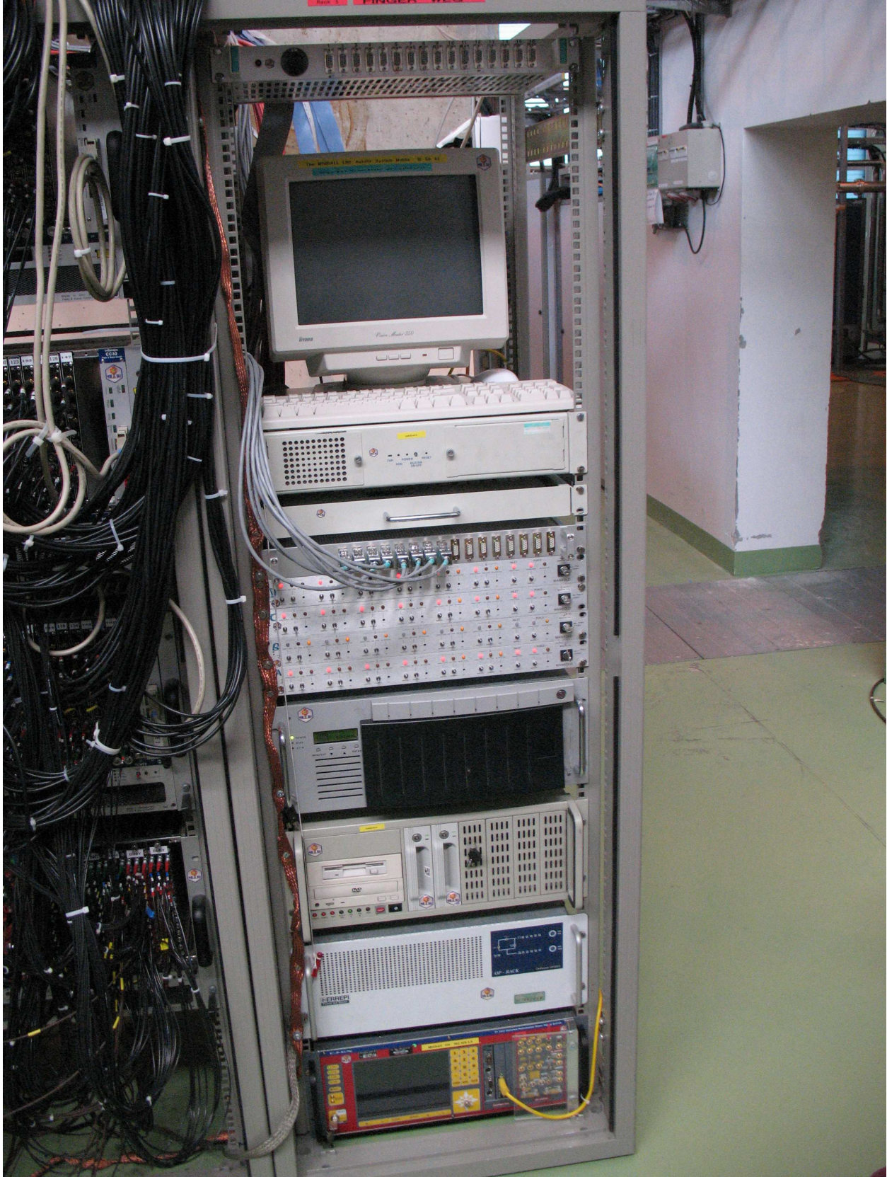
Figure 42: R5 bottom: filling system computer with monitor and keyboard, new PT100 box and four manifold controller boxes, raid array, DAQ computer, UPS, CAEN HV power supply. The old PT100 box is above the monitor.
