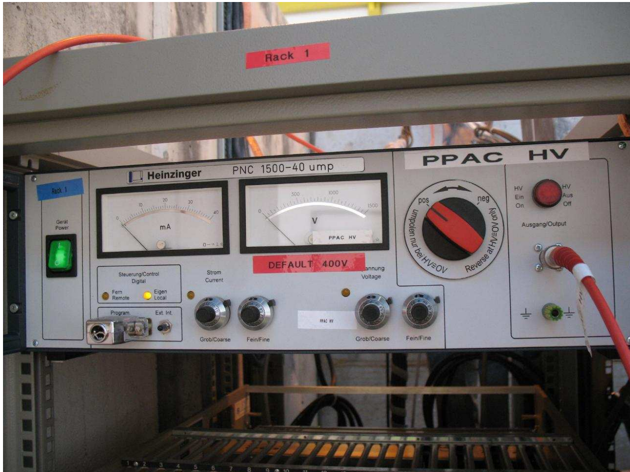
Figure 27: R1.C1: PPAC power supply. We normally use about +400 Volts
