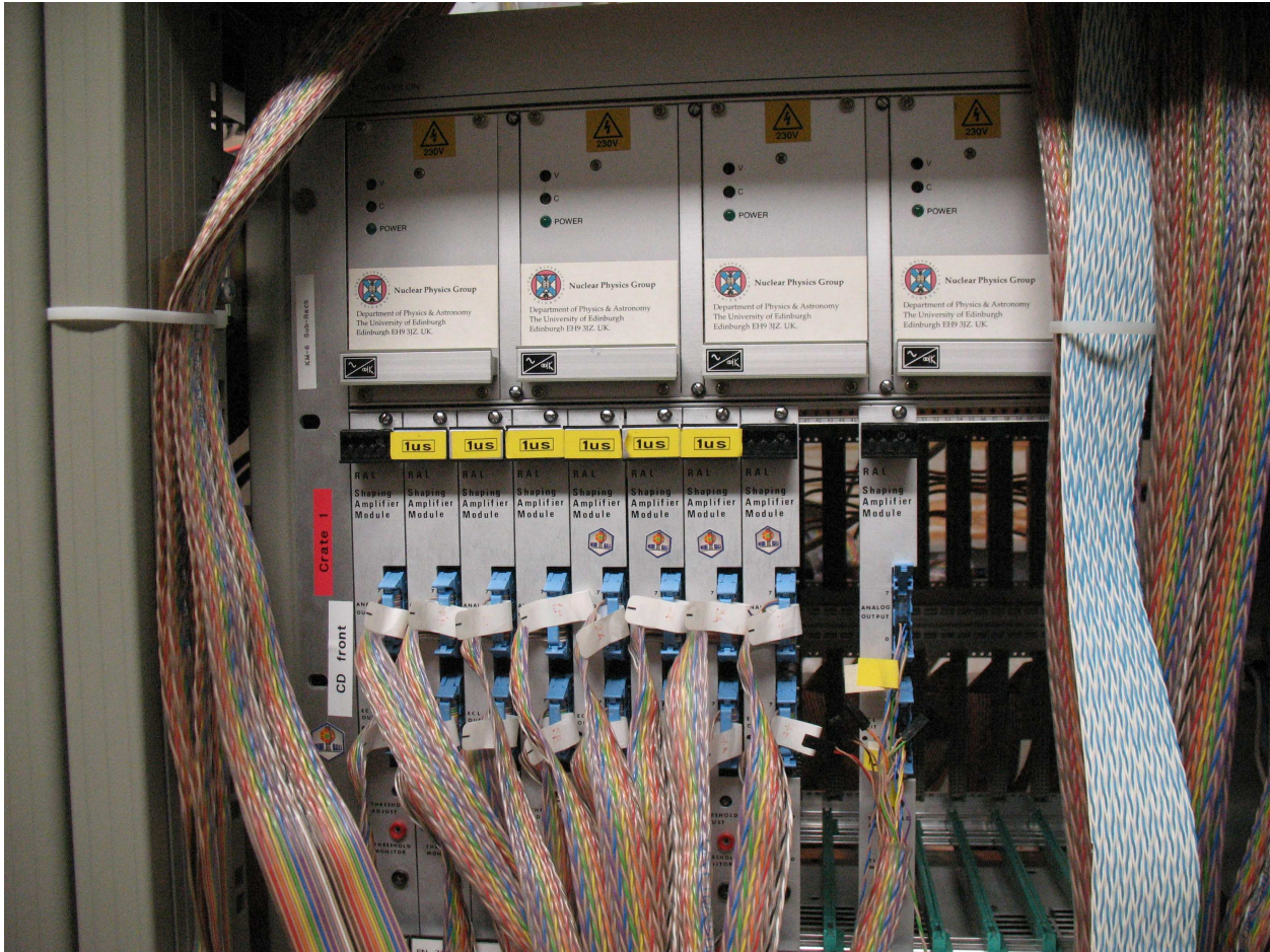
Figure 31: R2.C1: The RAL109s for the front rings. The upper connections are for the energy and they are joined up in pairs and sent to the ADC. The lower connections are for the timing and they go to the MALU in R1.C2 and from there to the TDCs in R3.C1.
