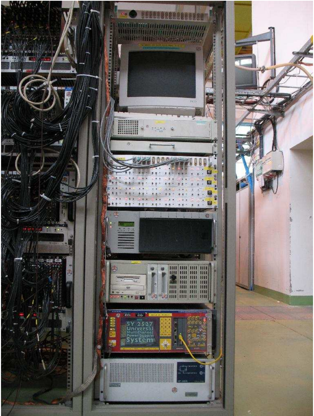
Figure 45: R5 bottom: filling system computer with monitor and keyboard, new PT100 box and four manifold controller boxes, raid array, DAQ computer, CAEN HV power supply and UPS. The old PT100 box is above the monitor.
