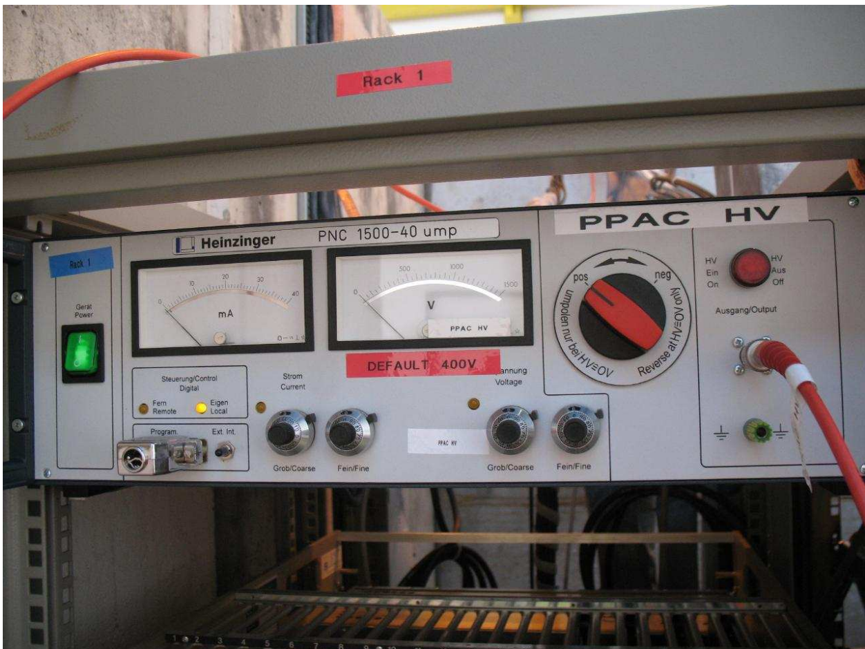
Figure 29: R1.C1: PPAC power supply. We normally use about +400 Volts
