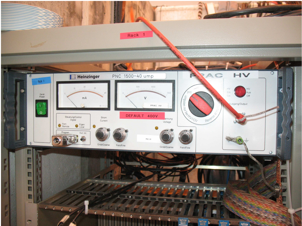
Figure 33: R1.C1: PPAC power supply. We normally use about +400 Volts
