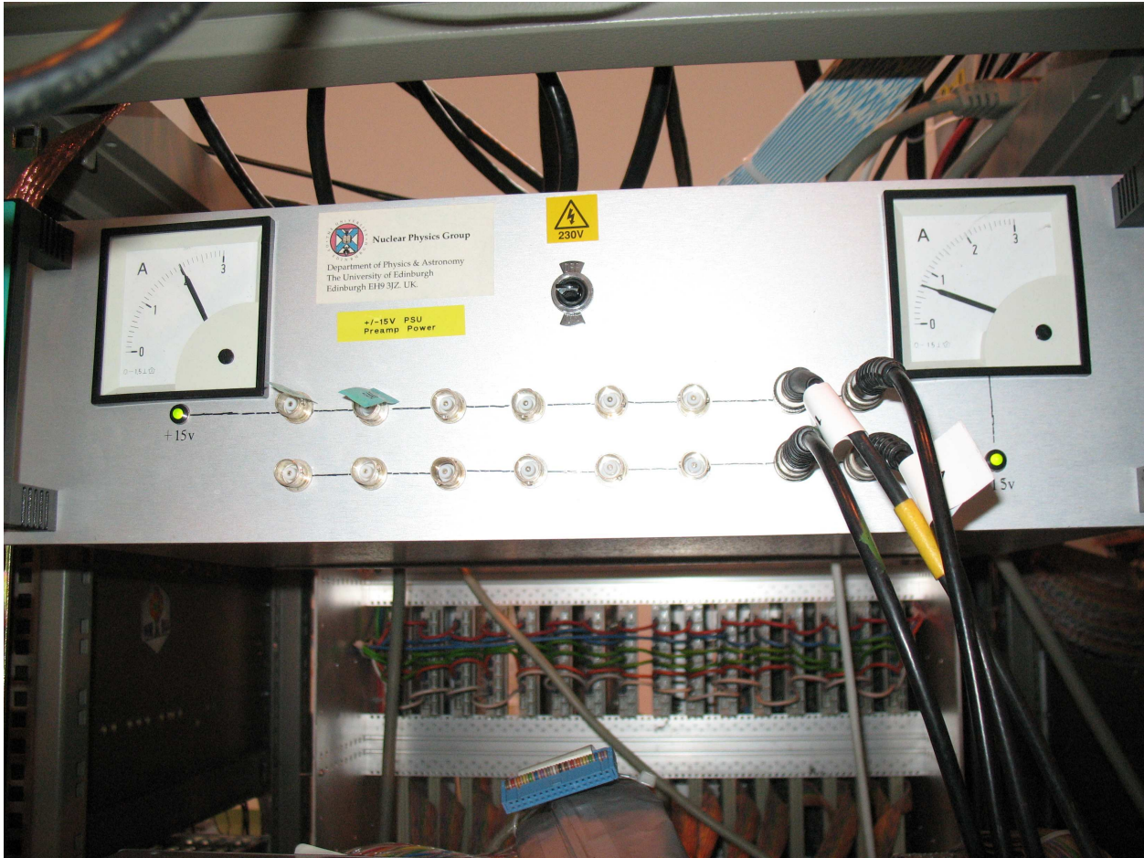
Figure 41: R2.rear: +/-15 Volt power supply for the CD preamps
